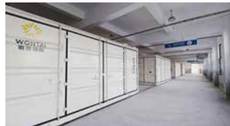
Wenzhou Hongfeng Electrical Alloy Energy Storage Power Station Project
