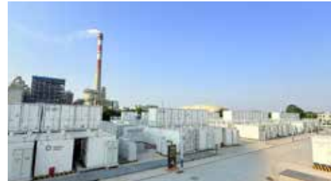
Energy Storage Project of a Power Plant in Hebei
