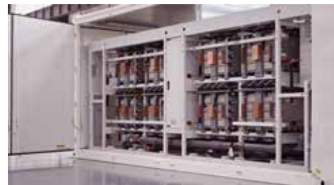
Guangzhou Modern Energy Storage Project An urban central park demonstration project
